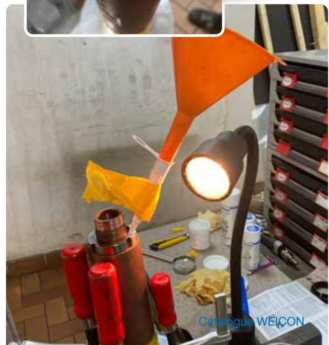
Interstitial grouting on a pipe-in-pipe system for electrical insulation | WEICON Casting Resin MS 1000
